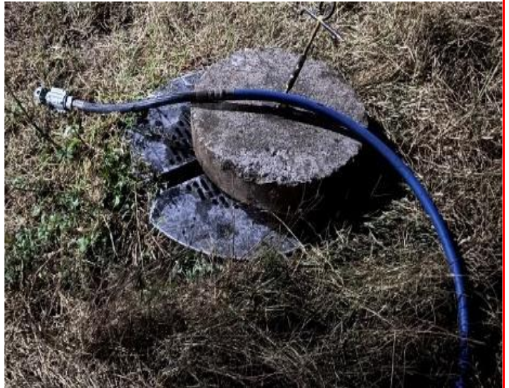
Hose, nozzle, grate and maintenance hole cover
